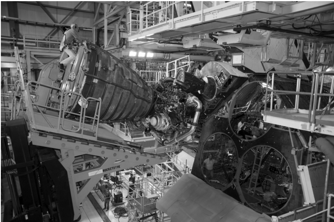
Figure C-41. A SSME lifted for installation into engine position No. 1 of Discovery , OPF-3, camera facing northwest, June 30, 2010.
